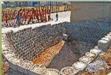
Storm water control
